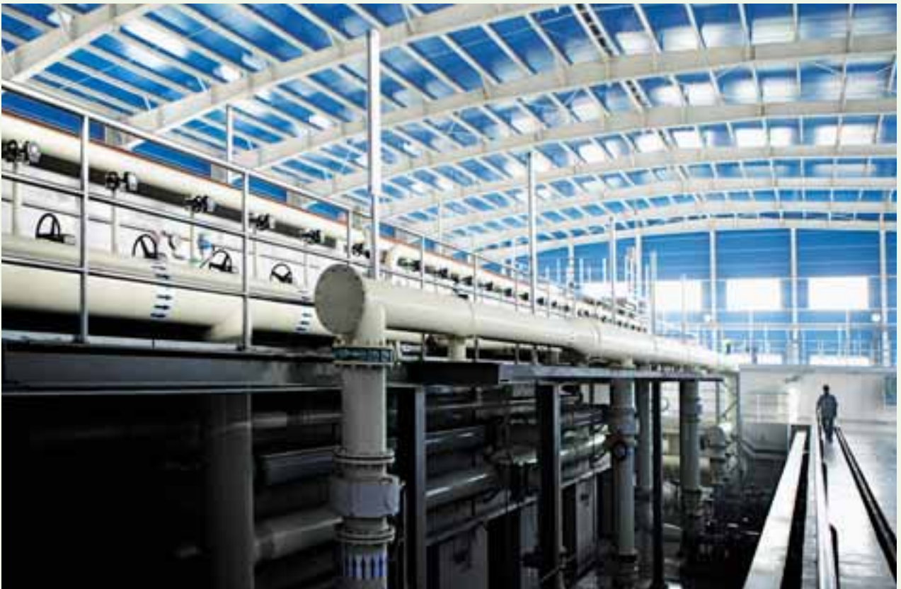
GE water purification facility in Beijing, China
